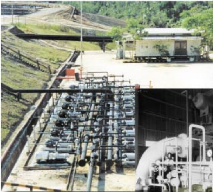
(16) 6D-312 pumps on crude oil pipeline service in the Pacific Rim area
